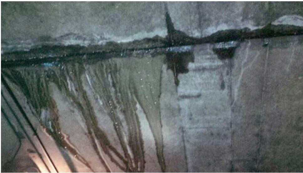
Leaking Tunnel Walls
