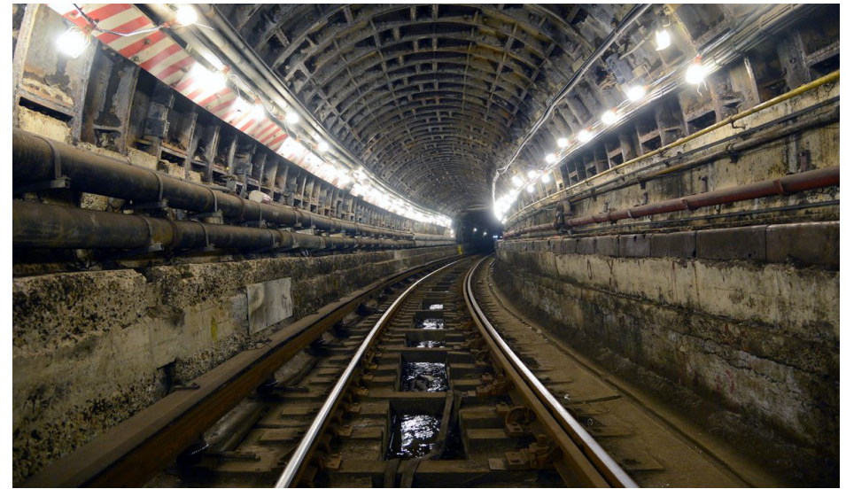
Standing Water in Tunnels
