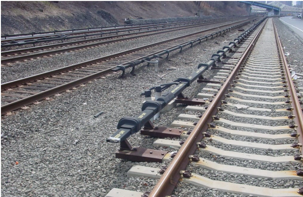
Third Rail (and associated components)
